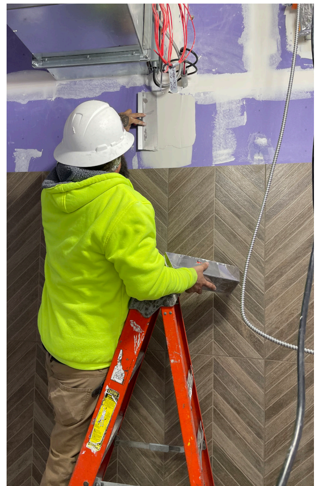
A worker joins drywall on the Heritage Center addition, with a peek at the herringbone accent panels in one of the new restrooms.
